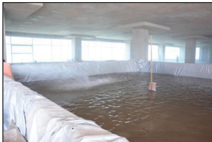
Fig. 8 Load testing on strengthened slab panel (Courtesy:- M/s R & M International Pvt Ltd)
