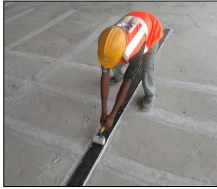
Fig.2 Application of Non prestressed FRP laminates in slabs (Courtesy:- M/s R & M International Pvt Ltd)
