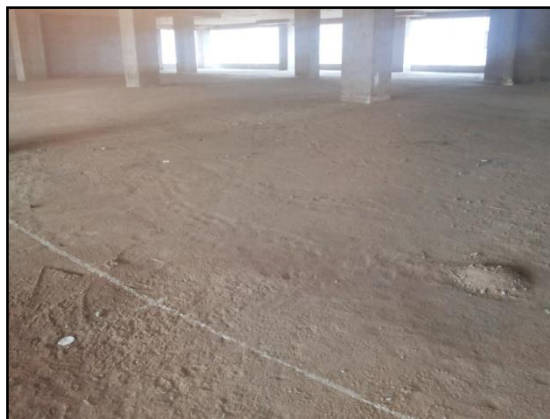
Fig. 6 Excessive deflections observed in midspan of flat slab panel (Courtesy:- M/s R & M International Pvt Ltd)
