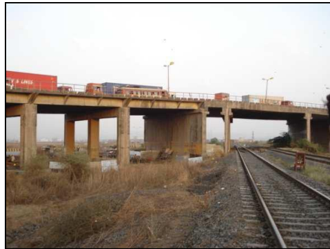
Fig. 9 Rail Over Bridge (ROB) at Karal junction of JNPT [9] (Courtesy:- M/s R & M International Pvt Ltd)
