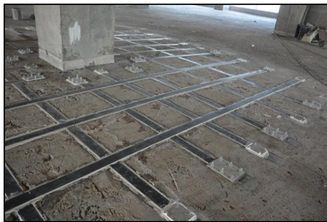
Fig.7 Application of Prestressed FRP laminates in slabs (Courtesy:- M/s R & M International Pvt Ltd)
