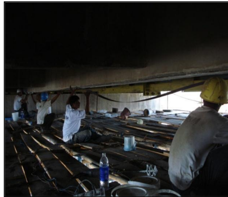
Fig. 10 Prestressing of CFRP laminates at bottom of girder [9] (Courtesy:- M/s R & M International Pvt Ltd)
