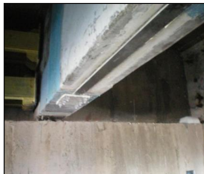
Fig. 11 Prestressed laminates with anchor plates at the ends [9] (Courtesy:- M/s R & M International Pvt Ltd)
